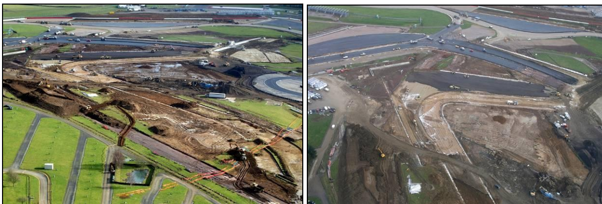
Work being carried out on the new Arena Grand Prix Circuit at Silverstone, scheduled for completion in March
